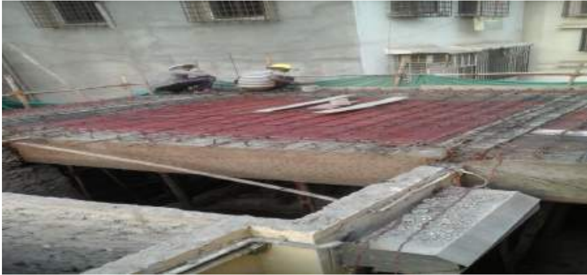
R J Market : Damaged Beam / Slab
